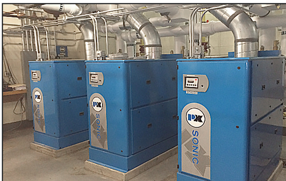
Heating units built by Harsco Industrial Patterson-Kelley and installed at the Elk Lake School District are expected to save the district millions of dollars.
